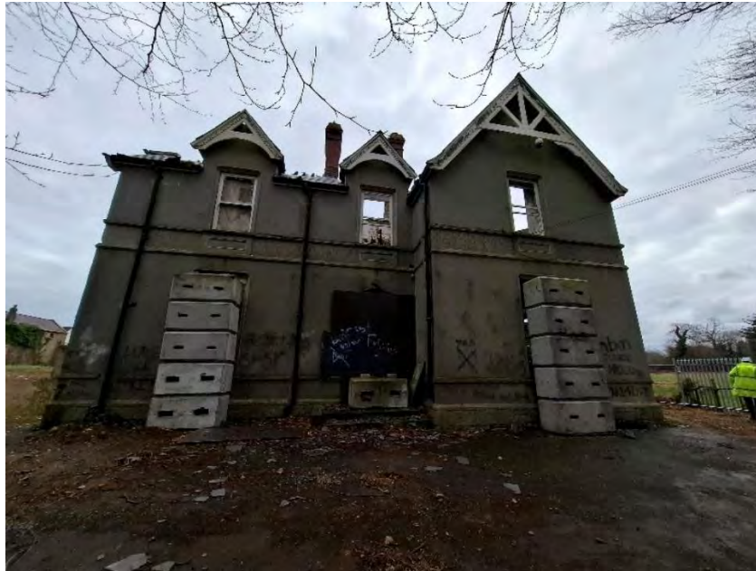
Photograph 6 - Northern facade. Windows demonstrate absence of ceilings/roof.
