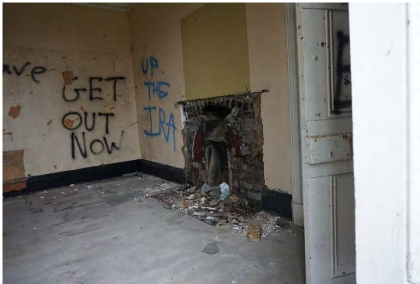
Photograph 13 - Fireplace features lost to fire.
