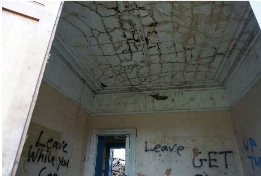
Photograph 12 - Water damage lath-and-plaster ceiling west facing room.
