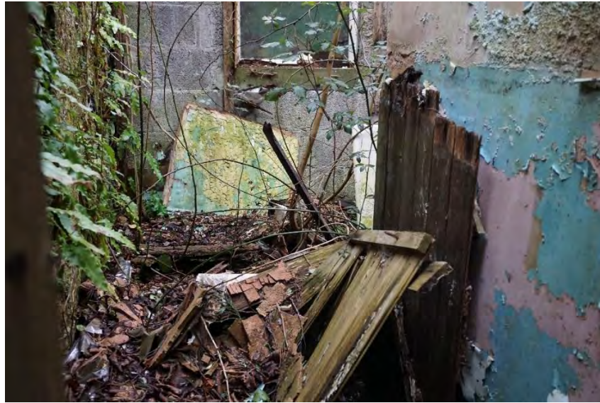
Photograph 18 - concrete blockwork extension to rear. Vegetation and signs of neglect.
