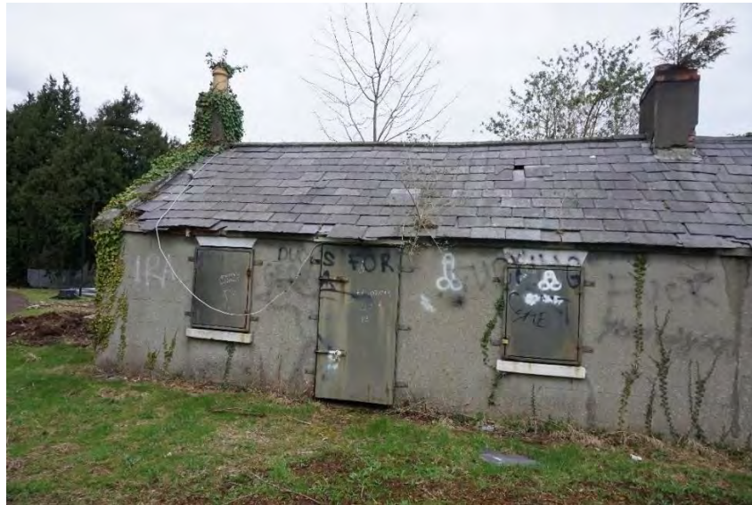
Photograph 14 - Gate Lodge front facade. Inappropriate modern interventions used over the years.
