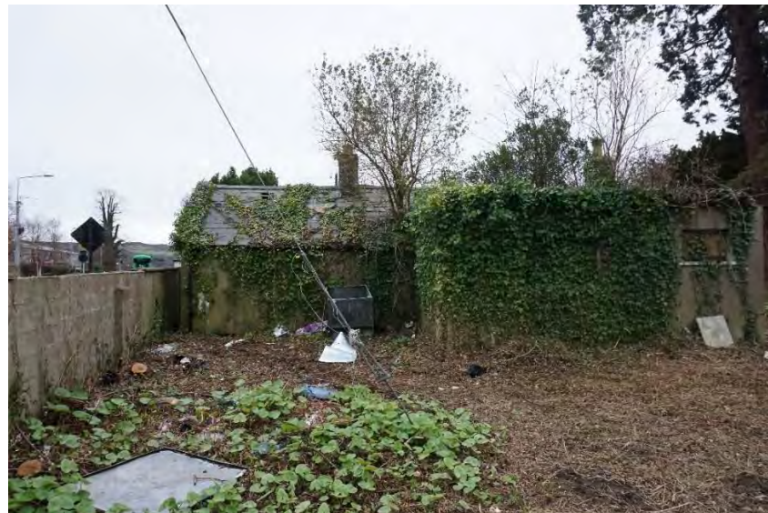
Photograph 15 - Rear Facade. Vegetation obscures true condition.
