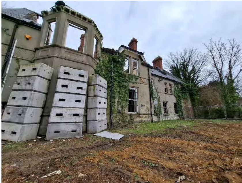
Photograph 8 - Rear facade from northwest. Rooms open to the sky.
