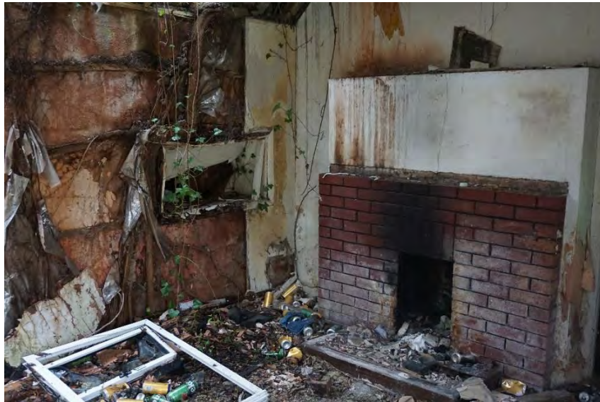
Photograph 16 - Debris, waste and modern interventions obscured much of the original fabric.
