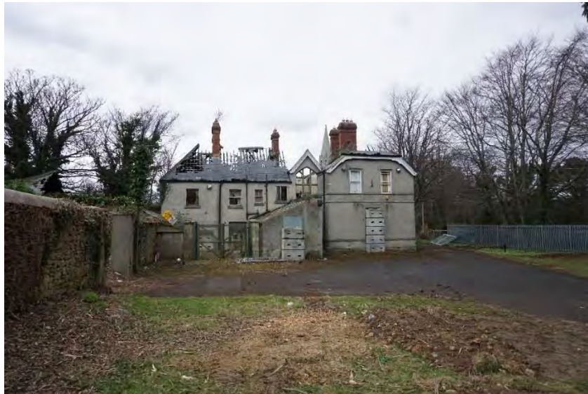
Photograph 2 - Roof damaged by fire.
