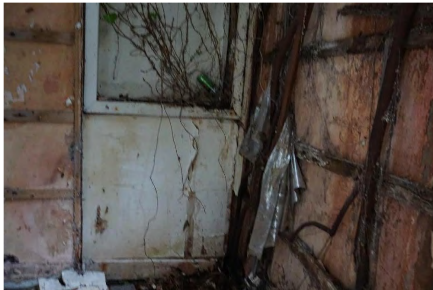
Photograph 17 - Indicators of moisture penetration and vegetation growth.
