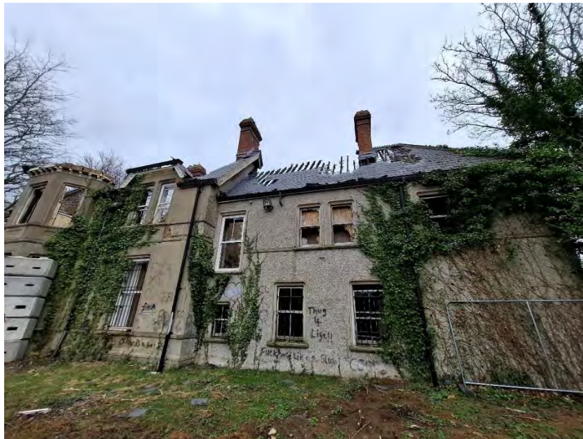
Photograph 9 - Rear facade taken from the southeast, open roof and partially boarded up window opes.
