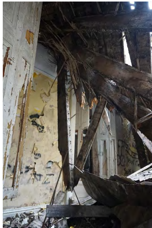
Photograph 11 - Room interior showing collapse ceiling joists.
